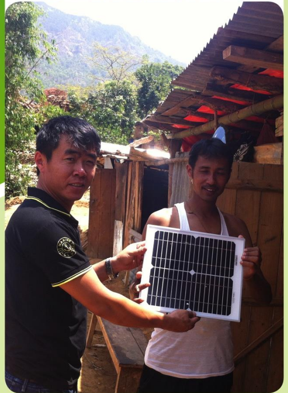
Nepal: This solar panel was installed at a temporary shelter in a village named Pipaldanda of Sindhupalchowk district, which was heavily affected from the earthquake of 25 th April 2015
