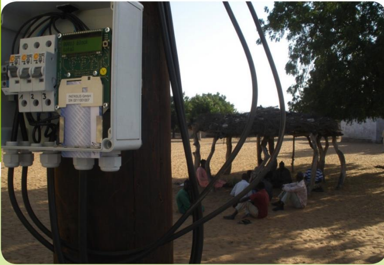
Senegal: Electrification of rural villages with systems operating on a fee-for-service basis
