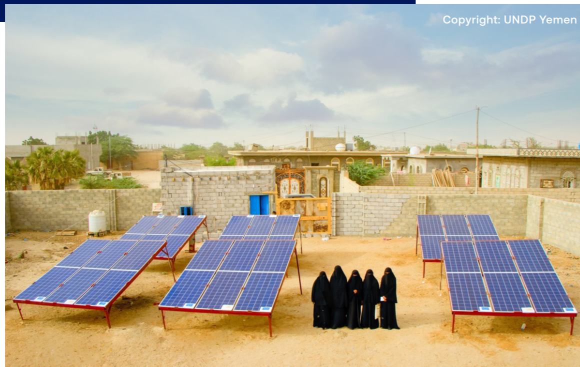
Figure 22. 63kWp mini-grid deployed in Hajjah, Yemen
