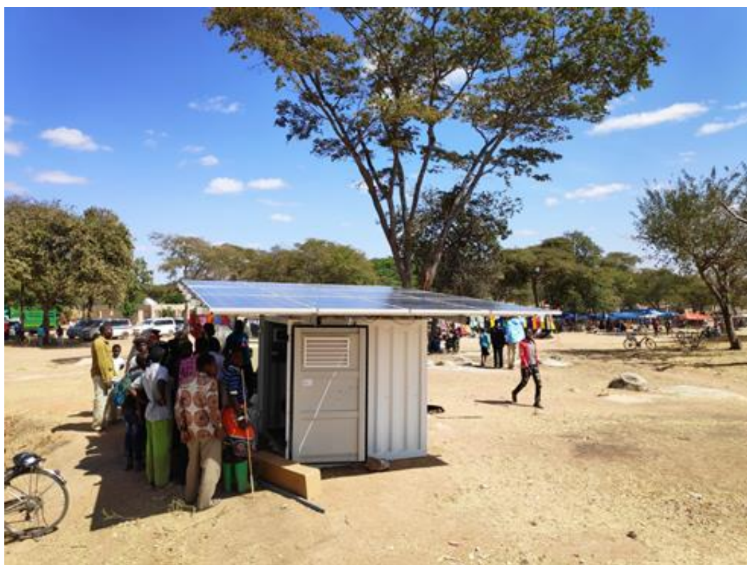
Off-Grid Box in Mtavira, Ikungi District, Tanzania,
