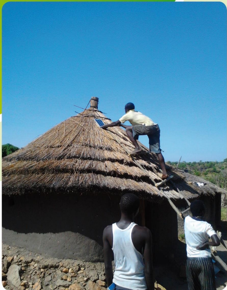
Uganda: installation of a solar panel on the roof of a hood. The PPP project 'Light Up A Village' in cooperation with Barefoot Power, uses picoPV to provide energy to the village of Fofo in the Moyo region, northern Uganda.
