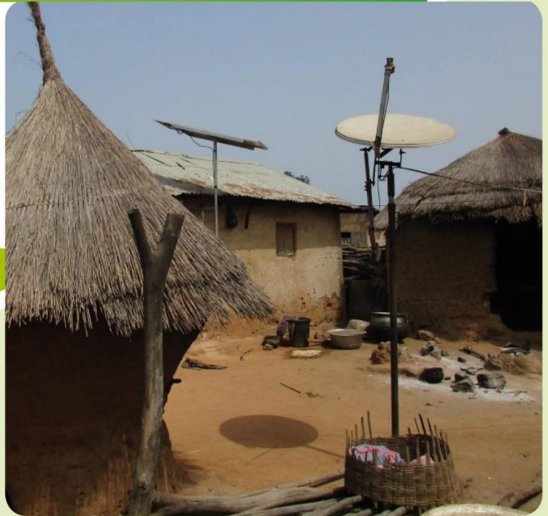
Benin: PV Solar Home System and a TV satellite dish on a family compound in rural Benin.
