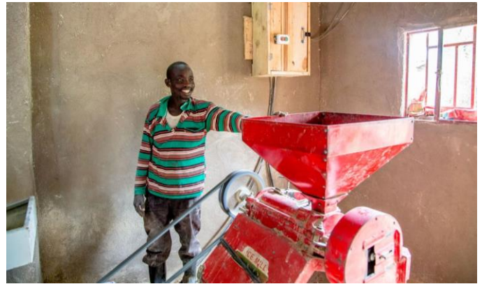
In Rwanda, entrepreneurs with access to solar energy are cutting costs and branching out.
